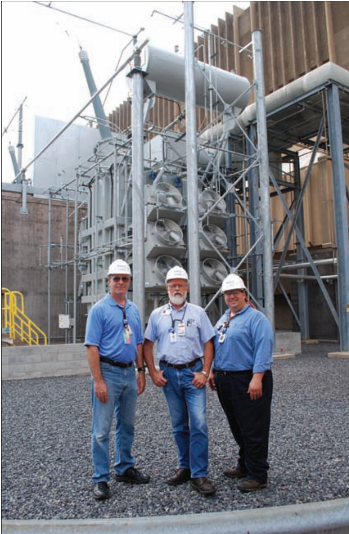
Limerick Generating Station replaced Limerick Unit 2's three main power transformers in spring 2011. Limerick's Unit 1's transformers will be replaced by 2016. Limerick employees are dedicated to operating the plant safely and reliably now and into the future.
