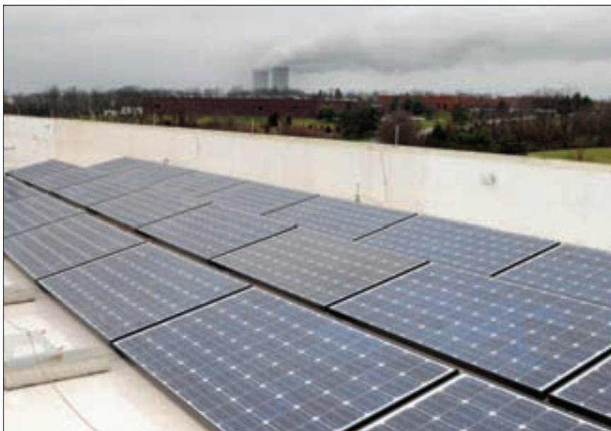
The solar panels installed by Helio Power Systems will provide the hospital with 88 megawatts of solar electric power.
